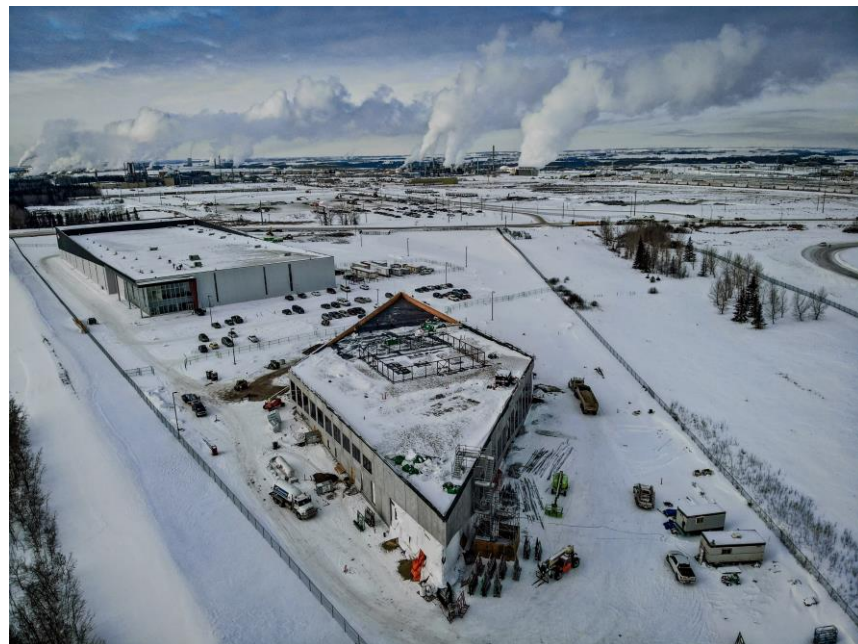
Diamond Centre – offices, workstations & meeting rooms ~65,000 sq ft (total building size) Includes 200-person auditorium
